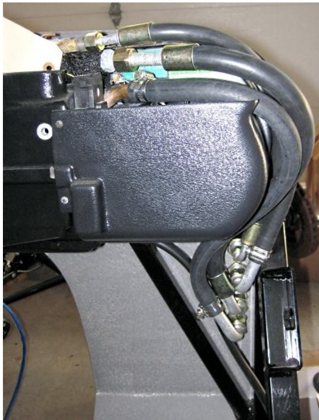
Route the hose down to the firewall and attach with a \frac{5}{16} " socket.
