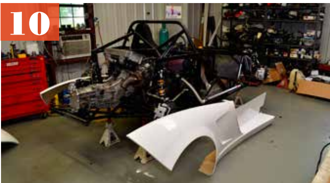
10 Most projects start at the beginning, but the body assembly process starts in the middle: The sides of our 818 would be the first components installed. Notice that everything comes in a nice, glossy white gelcoat—we won't have to paint the 818 when it's finished.
