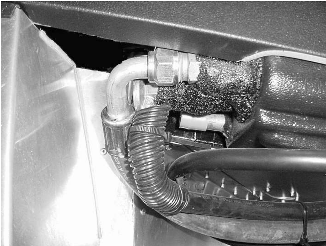
Pressure hoses attached to A/C evaporator. Note bottom edge of dash is trimmed for A/C fitment.
