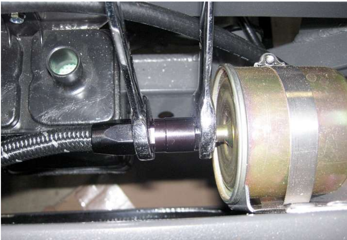
Tighten the end of the fitting onto the hose using 1\frac{1}{16} " and \frac{3}{4} " wrenches.
